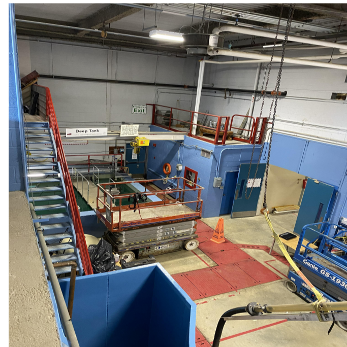
IMAGE 11: DEEP TANK AND EN-1035A
